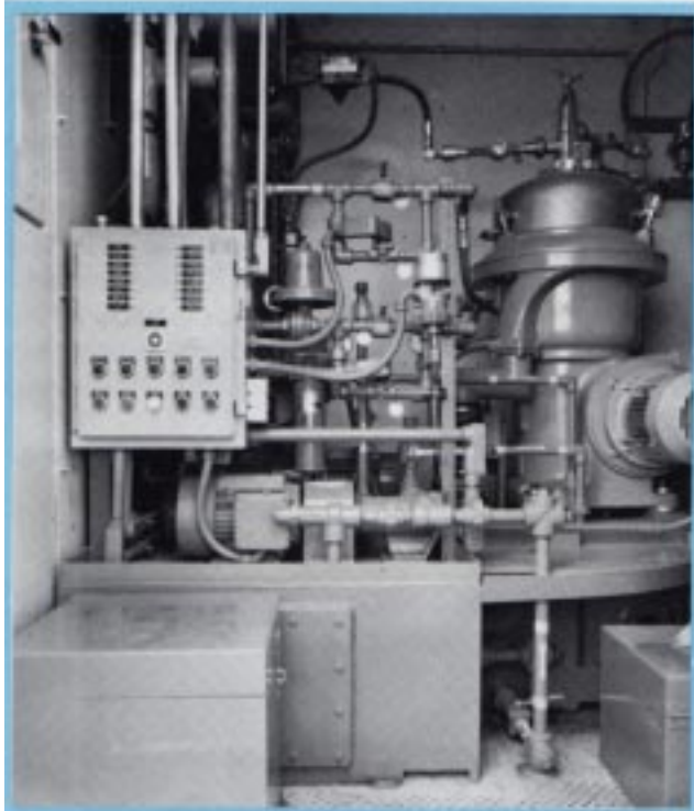
Centrifuge & Storage Tank
