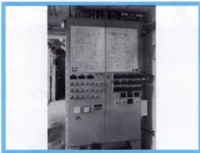
Control Panel in Lab
